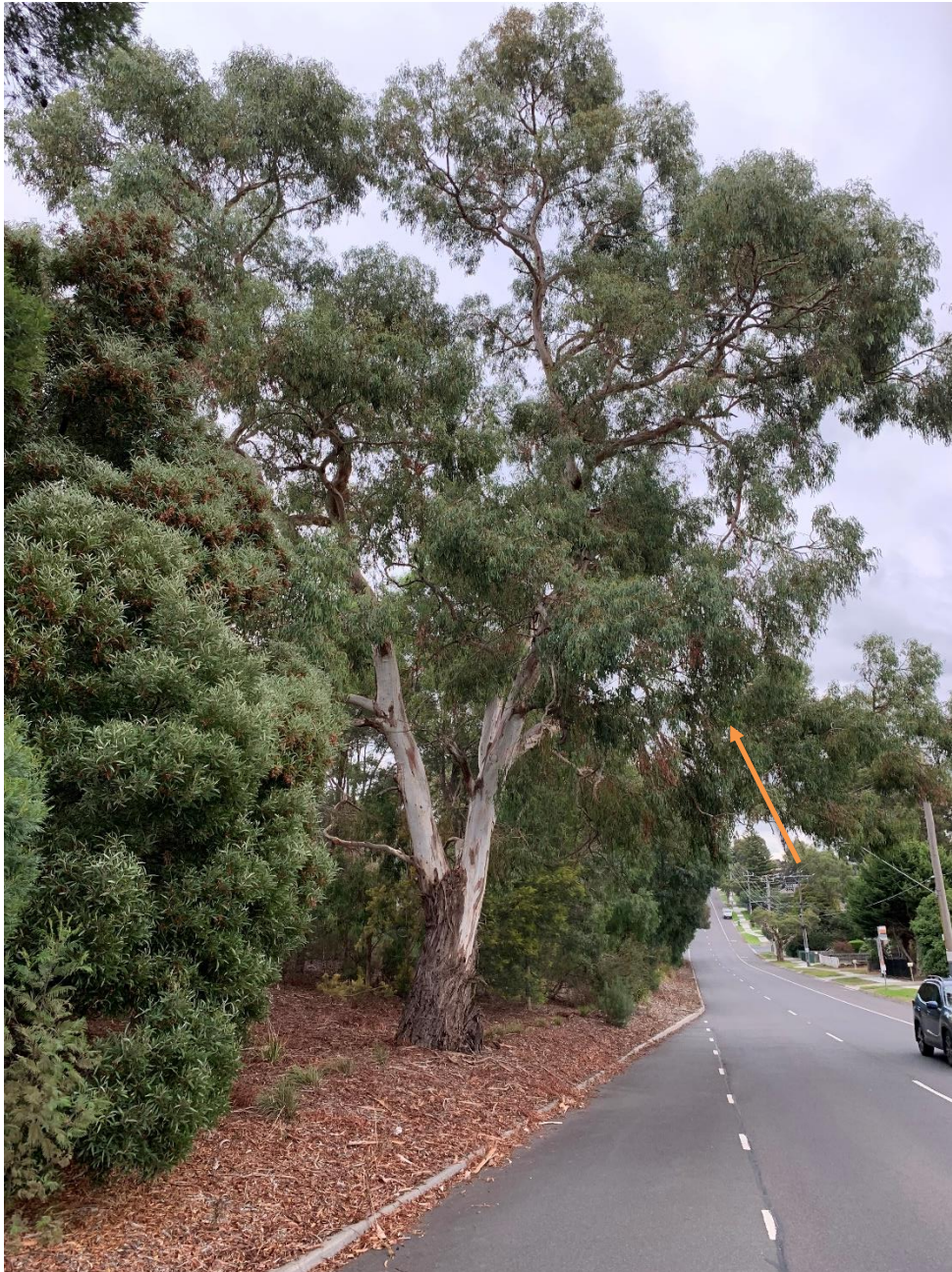
Tree 104 – This tree will have to be removed according to the current plans. The arrowed branch is at high risk of collapse onto the road.
